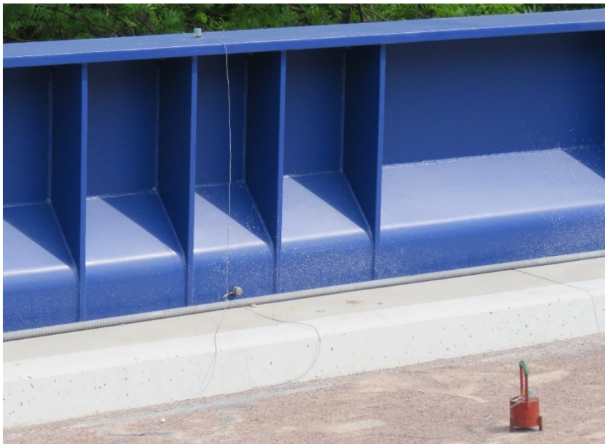
Figure 4. The view on the three accelerometers of type 8344 placed on the main girder and on the roadway.
