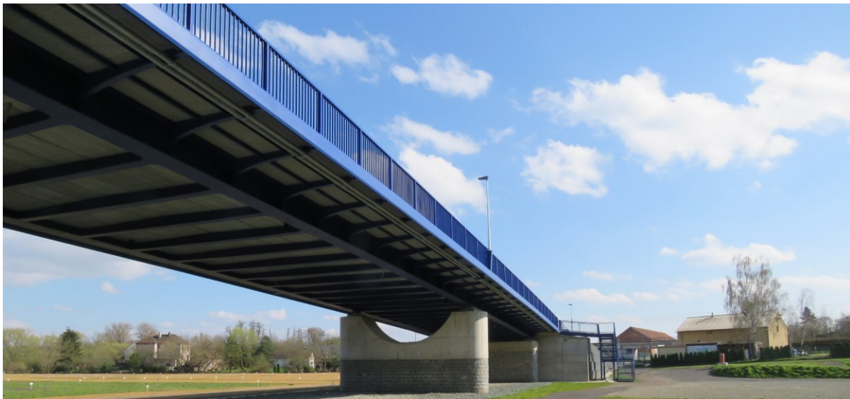
Figure 2. The bottom view on the load bearing structure in the second and first span of the bridge.
