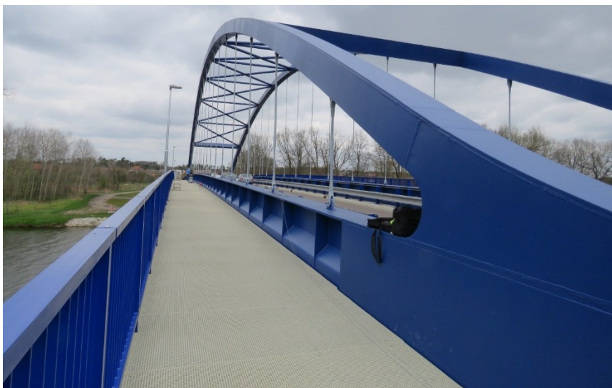
Figure 3. The view on the load bearing structure in the third span of the bridge.
